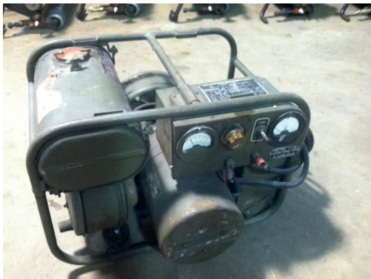
Figure 2. A typical small gasoline generator US GE-12-G from WW2. It has a 0.5 kW air-cooled 2-stroke 2-cylinder engine and produces 12 volts DC. [5: 572]
